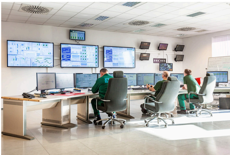
Thanks to Adasa's Insygnia solution, control room operators spend their time planning, supervising and monitoring standards and processes.
