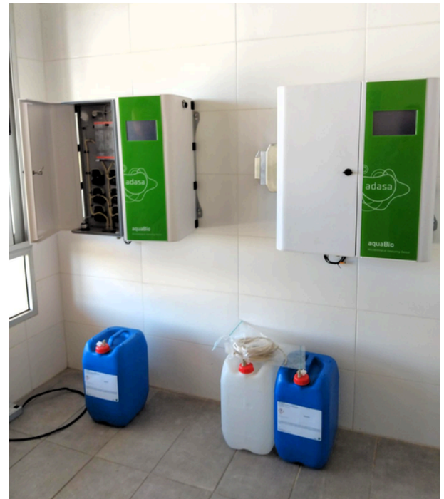
aquaBio systems installed in Montevideo, Uruguay.
